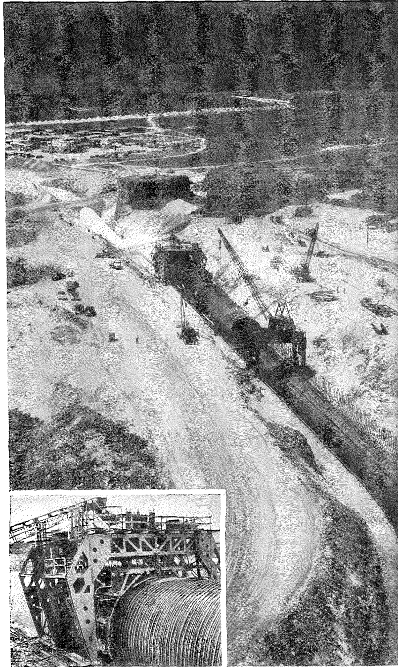
SIPHON WITH A STEEL THROAT. Extending around the north end of Soap Lake in the Grand Coulee area, this huge siphon, more than 22 feet in diameter, will carry irrigation water from an elevation of 1320 feet down into a 215-foot dip in the land's profile, and up again to an elevation of 1301 feet. The siphon is steel-lined concrete pipe. The 3400 tons of steel plate used to fabricate the liner sections were supplied by U.S. Steel, while the outside traveler and form (inset) and the inside traveler and collapsible ribs, were especially fabricated by U.S. Steel for the casting of this large conduit.
