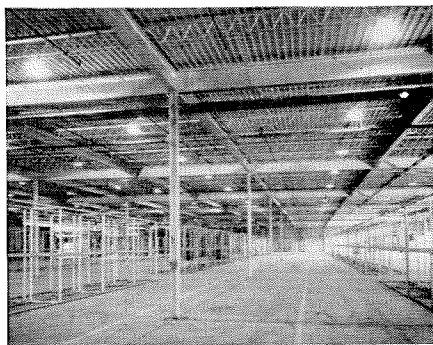
Fig. 1. Process warehouse for the Hale-Halsell Grocery Co., Tulsa, Oklahoma. Size 250' x 350' with 16' clear height. Contractor: Tulsa Rig and Reel and Manufacturing Co. Consulting Engineer: David R. Graham & Associates, Tulsa, Oklahoma.
