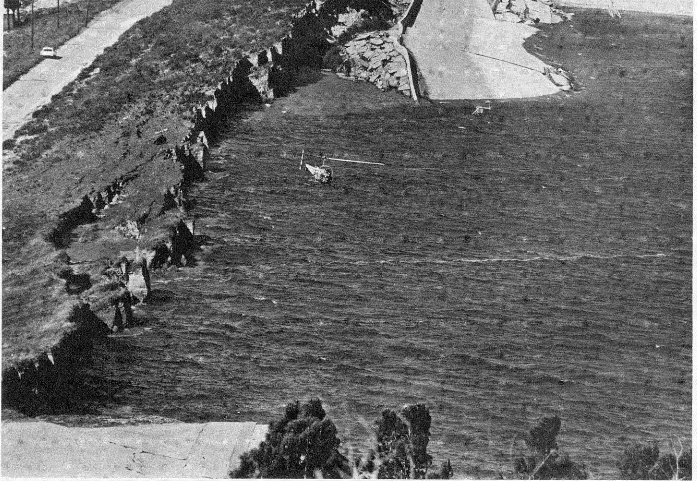
The luckiest feature of this earthquake was the survival of the lower Van Norman dam—which looked like this on the morning of the quake. A major section of the dam slid into the reservoir, leaving a scarp of about five feet between the water level and the top of the remaining portion of the dam.
