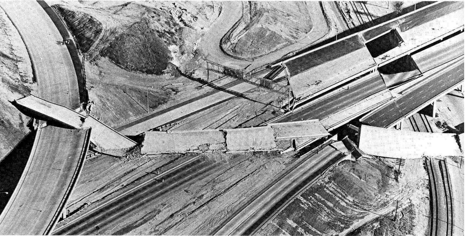
This is one good reason why earthquake engineers feel there are many improvements that can be made in highway structures. Nearly every bridge and overpass structure in the interchange between the Foothill and Golden State freeways was seriously damaged by the earthquake.
