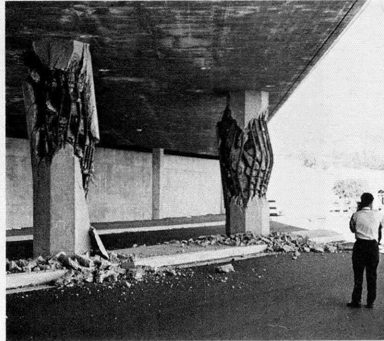
Columns on the Foothill Boulevard overcrossing of the Foothill Freeway were severely damaged. The complex failure of the bridge was aggravated by the inadequacy of the 1/2-inch horizontal ties that were supposed to confine the 2 1/4-inch-diameter vertical reinforcing steel.
