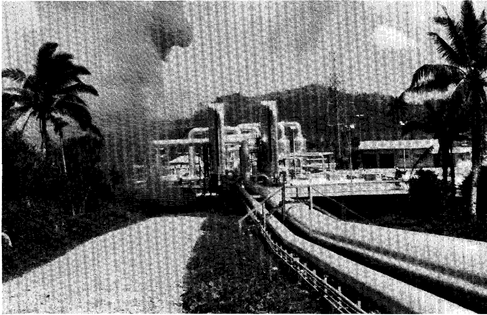
High- and low-pressure steam pipelines carry geothermal energy to a power plant in Tiwi, Philippines, equipped with a double inlet turbine; the scrubbers in the background eliminate moisture and dissolved constituents from the steam before delivery to the plant.
