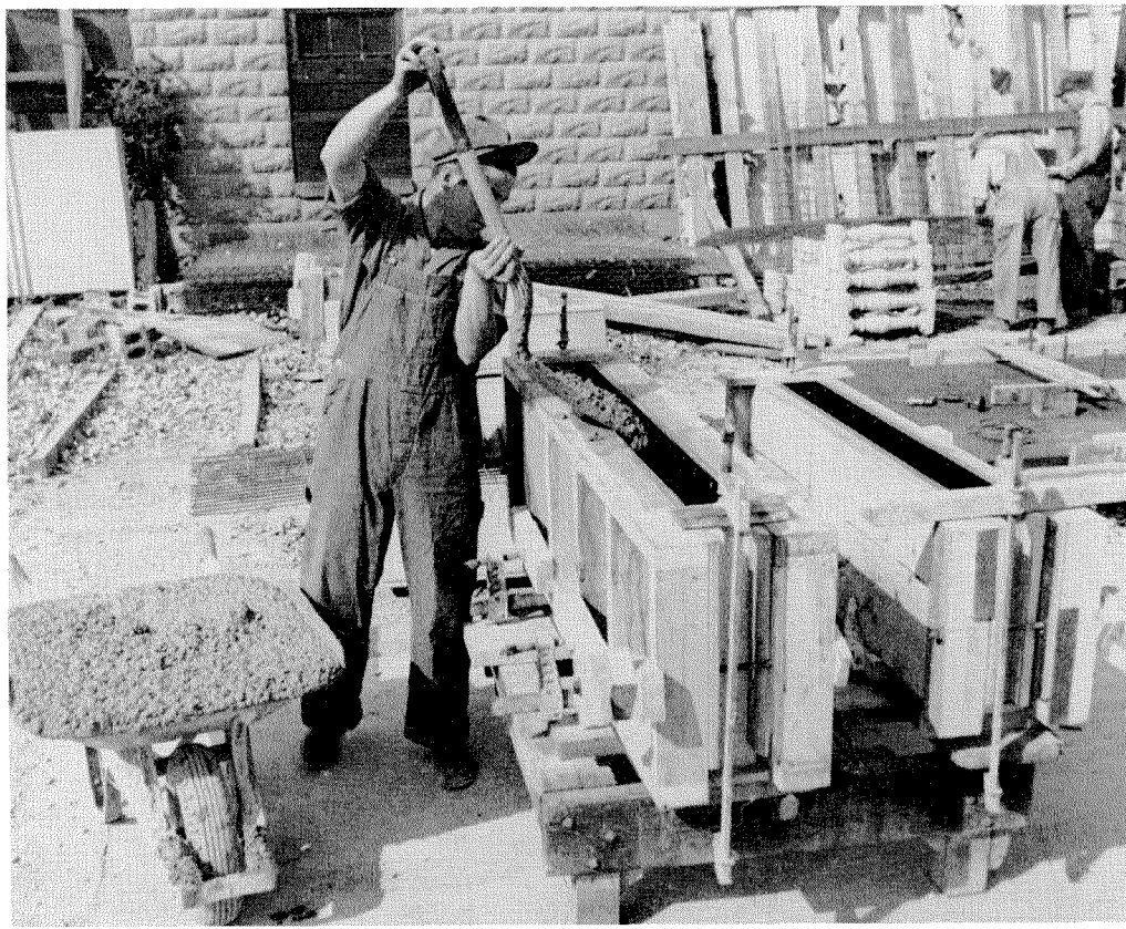
"Kimpreg" surfaced plywood used for the manufacture of pre-cast stone. These forms will withstand in excess of 100 casting operations. Courtesy of the Kimberly-Clark Corporation.
