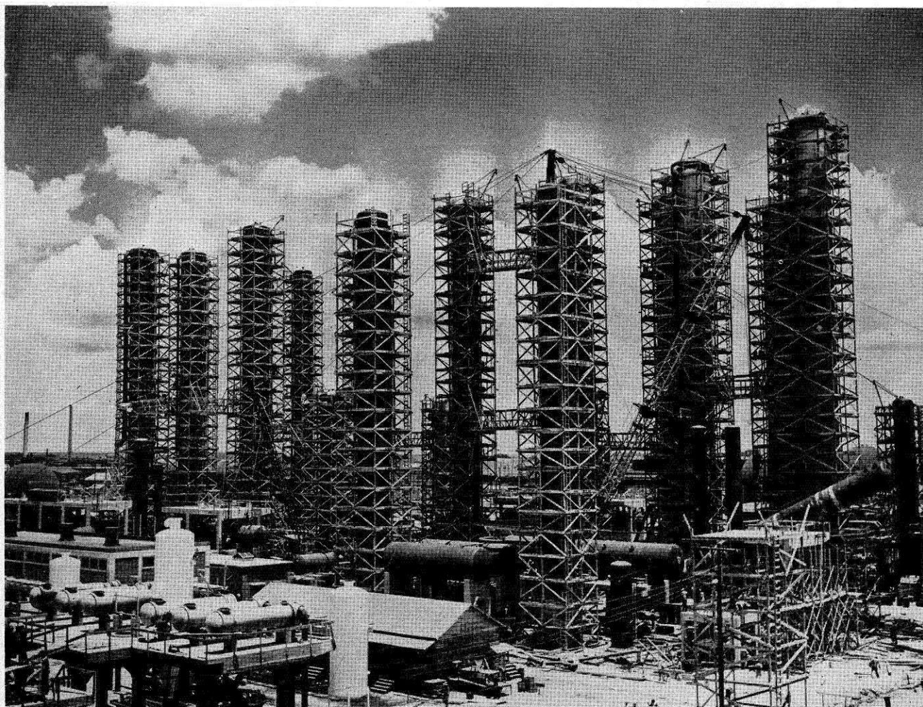
View of large towers under construction for butadiene plant, showing method of erection.
