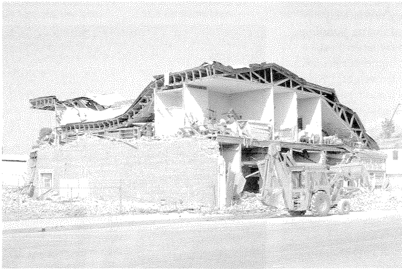
Above: This unreinforced masonry building in downtown Coalinga collapsed in the 1983 earthquake. Many California cities still have large stocks of such buildings, and no retrofit programs.
