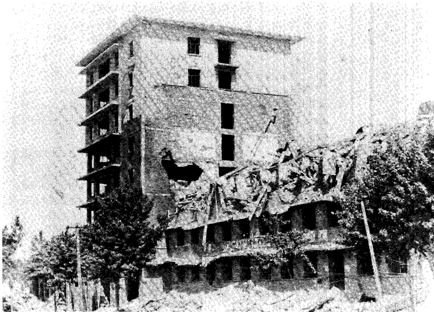
The eight-story Hsin-Hua Hotel was badly damaged at the fifth-story level, but it remained standing. In the foreground is a six-story building that collapsed completely. The behavior of soft soil had an appreciable effect on the damage sustained by structures; that is, buildings located on thin soil, on thin layers of rock, or on thin layers of soil over rock did not exhibit the same degree of severe damage as buildings located on less firm soil.
