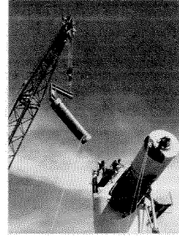
Right: It took three cranes, manned by a rigging crew of 12, to lift one of the huge dishes onto its pedestal. Securing it in position involved meshing the pedestal gears with the driving gears on the dish, and welding two counterweights of 18 tons each onto the dish before the cranes could release their grip.
