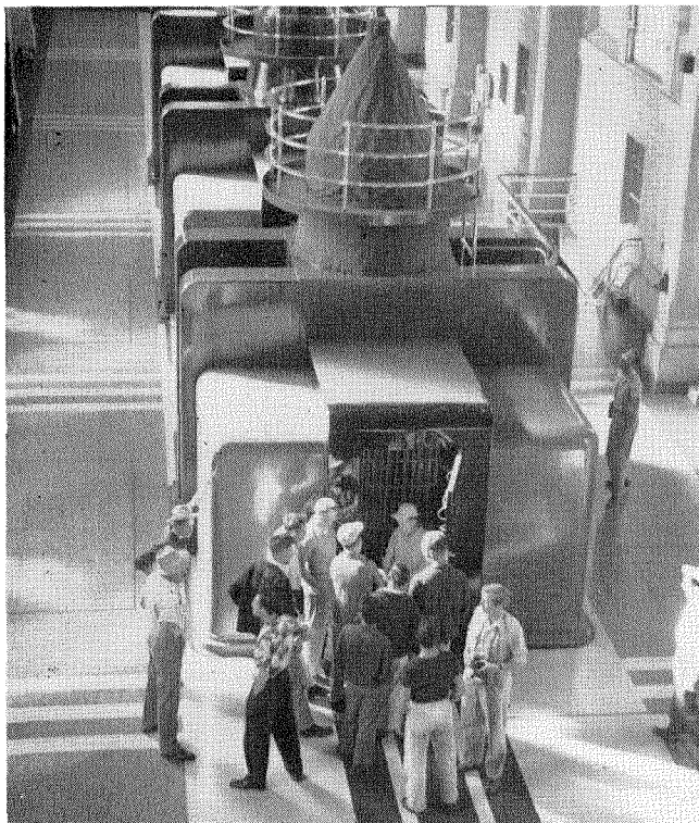
Inspecting pumps in the Gene Pumping Plant of the Metropolitan Water District.
