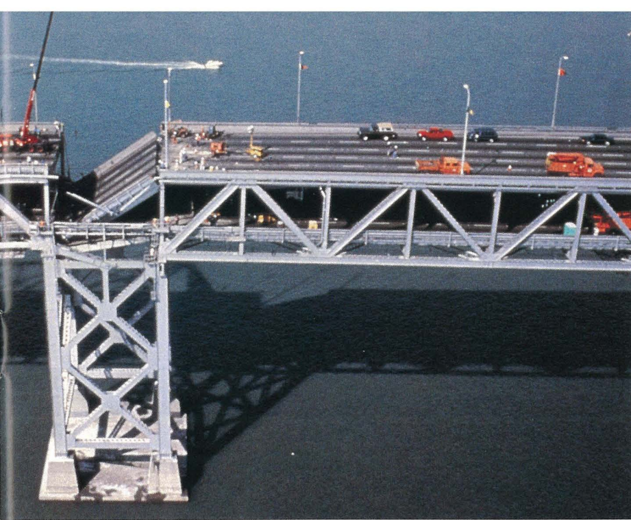
50-foot upper- and lower-deck spans of the Bay Bridge collapsed across a pier when shaking broke loose one truss to which the decks were attached, resulting in a 7-inch movement toward the Oakland side, which pulled the decks off their seat supports on the San Francisco side.
