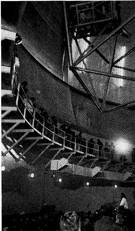
Right: Under the telescope's secondary-mirror cage, Silva chants the invocation. The ductwork below the catwalk is part of an air-handling system that can replace the entire volume of air inside the dome with outside air every five minutes. This prevents electrical equipment (and humans) from heating the dome air, making it unstable.
