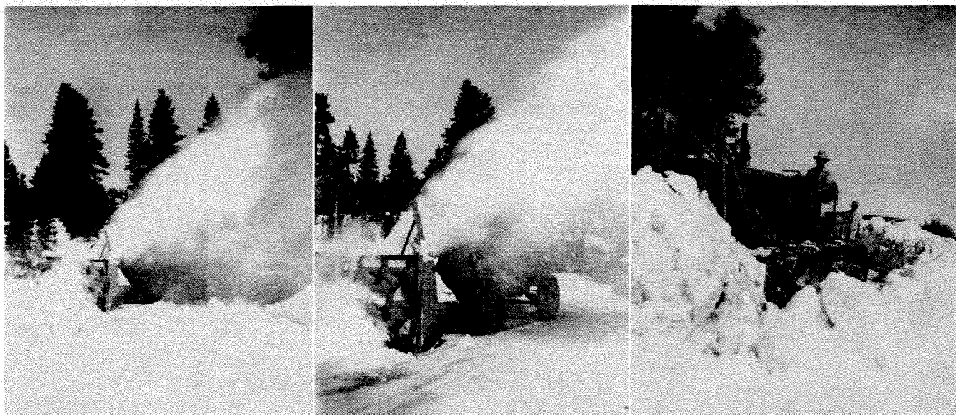
FIG. 1. (Left) Rotary snow plow in action—Big Pines Road. FIG. 2. (Center) Another view of the rotary snow plow in action—Big Pines Road. FIG. 3. (Right) Bulldozer on Mt. Wilson, March, 1944.
